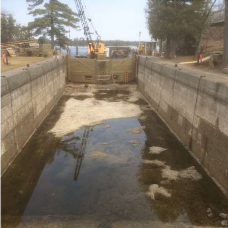
Log replacement lock 30 Spring 2014
